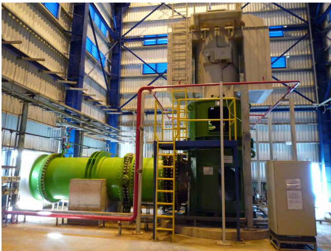
Main Cooling Water Pumps
