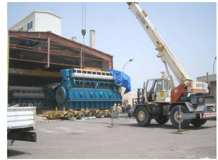
Installation of a 10.5 MVA power generator
