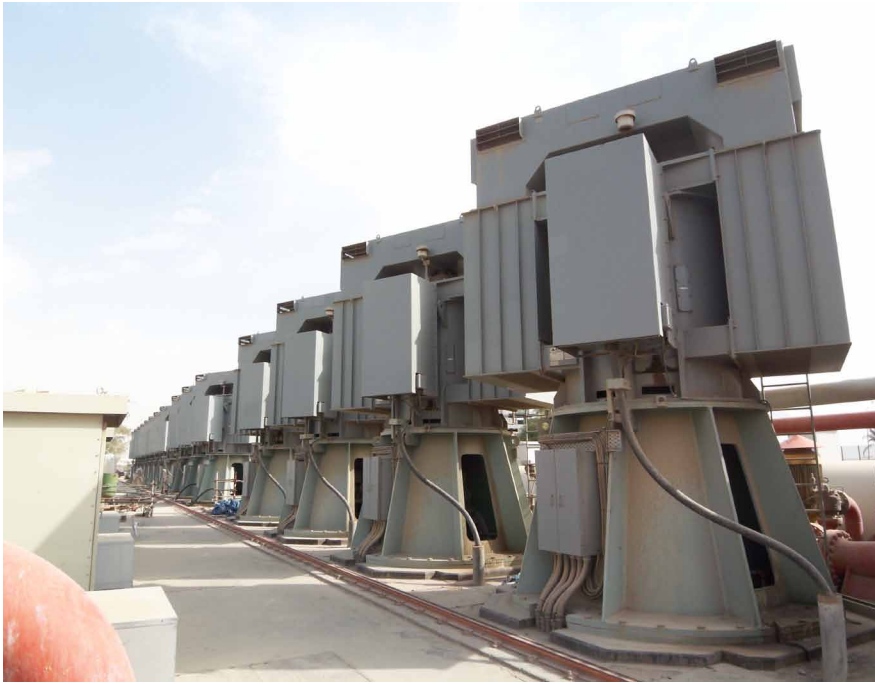
Supply Cooling Water Pumps
