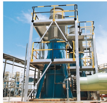
Sea water cooling pumps, Singapore (Size:800mm, Driver:790kW)
