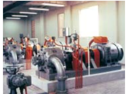
Distributing pumps in small-capacity water works
