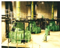
Sewage pumps (size : 1300 × 1100mm), Hong Kong
