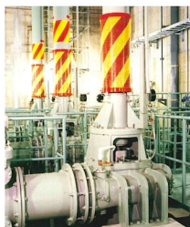
Sewage pumps (size : 450mm), Japan
