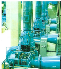
Intake pumps in city water plant (size : 800m), Hong Kong
