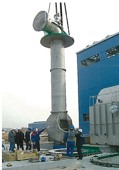
Hot well pump for Germencik Geothermal power project, Turkey (Size : 1000mm, Driver : 600kW)
