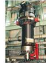
Boiler circulating pump (Pusan Combined Cycle Power Station)
