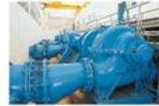
Distribution pump (Patat Gedde Pump Station, Surabaya)
