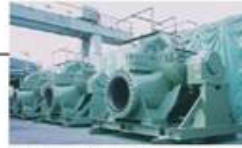
Double suction drinking water transmitting pump with high total head 250m (Shawwat Water Transmission Scheme)
