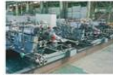
Ring section B.F.P. (Iran Power Plant Management Company)
