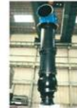
Discharge pump (Chang Water Reclamation Plant)
