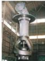
Hot well pump (Olkaria Geothermal Power Plant)
