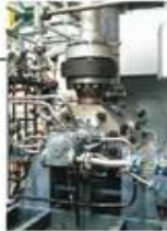
Ring section B.F.P. (Fujairah Water and Power Plant)
