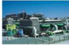
Various seawater pumps in the MSF desalination plant (Al-taweelah A2 Desalination Plant (Al-taweelah B Desalination Plant))
