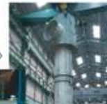
Circulating water pump
