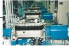
High pressure pump for RO desalination plant (Jeddah)
