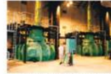
Vertical sewage pumps in the biggest sewage plant in Asia (Stone Cutter Pumping Station, Hong Kong)
